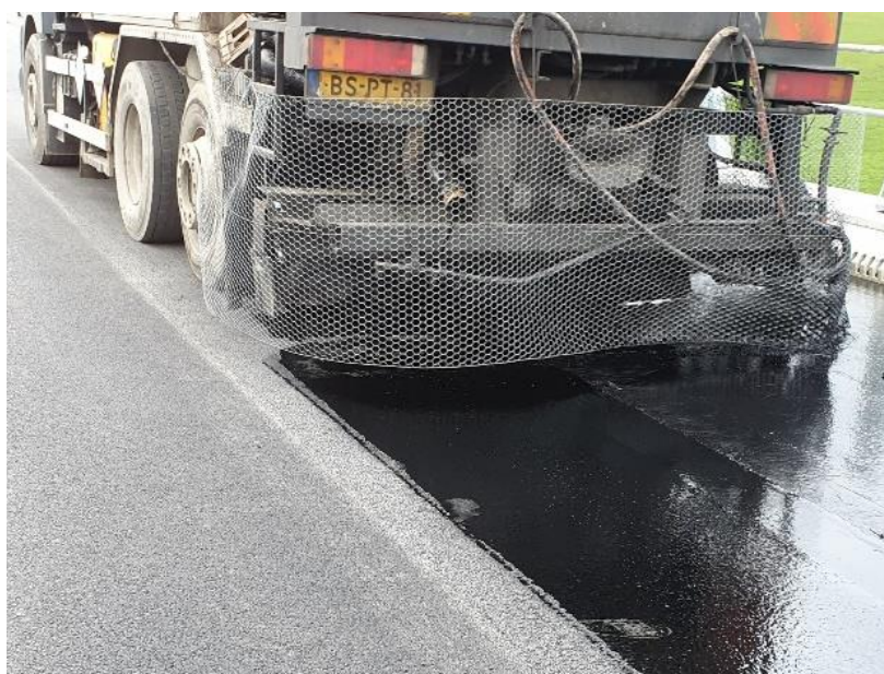
Figure 12: Applying adhesive layer and protection method for removal of cobwebbing effect resulting from high winds on site.
