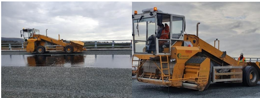
Figures 13 and 14: A Phoenix forward spreader was used to apply 10mm chippings to the PMB bitumen membrane once curing had taken place (within 30 minutes to 1 hour after spraying).
